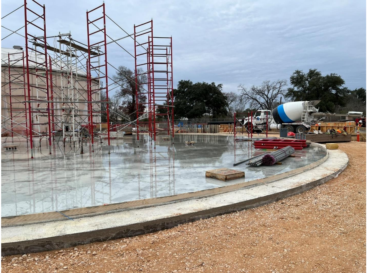
2H - Ground level view (b) of Tank Floor Structure, including water stop material at Floor perimeter.
