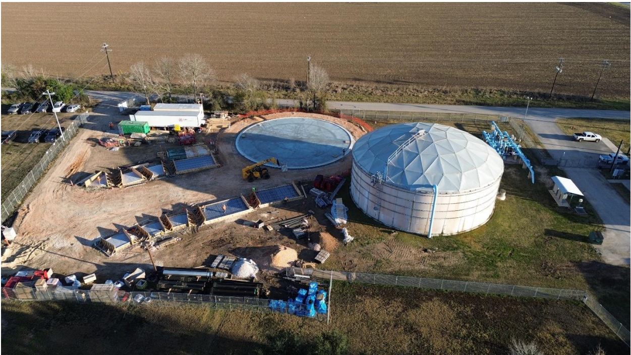
2D – Aerial side view of completed concrete pour at Tank Floor Structure.
