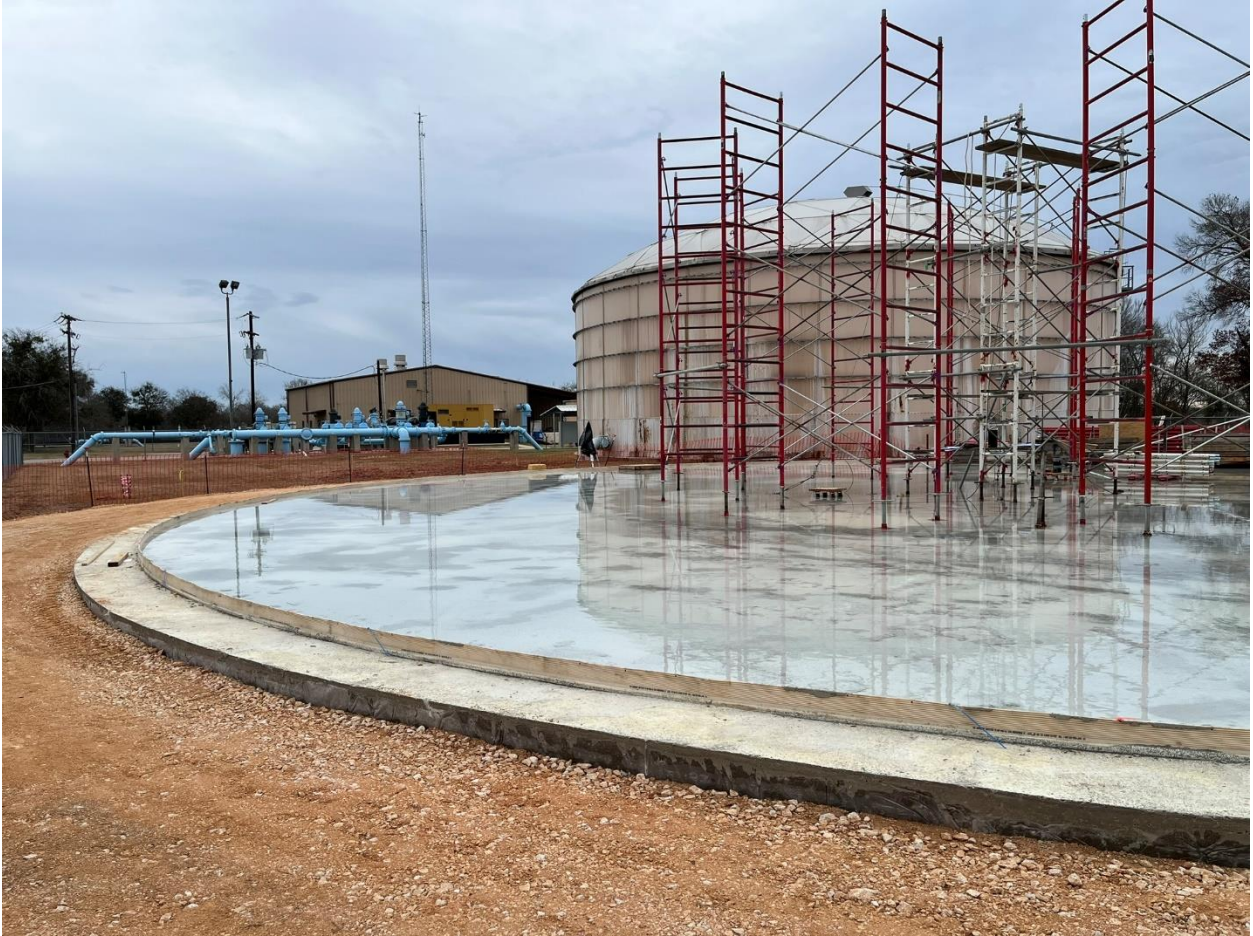
2G – Ground level view (a) of Tank Floor Structure, including water stop material at Floor perimeter.
