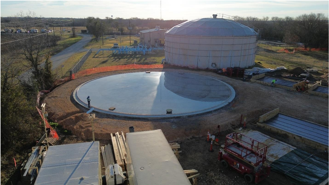
2E – Aerial side view of completed concrete pour at Tank Floor Structure (submerged in water for cure).
