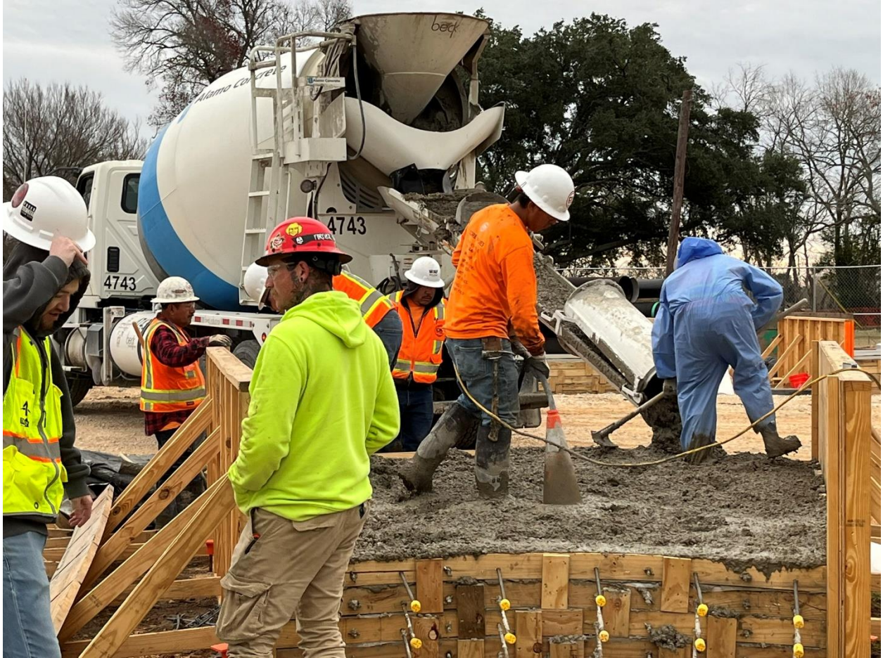
2M – Spreading and vibration of concrete at reinforced Dome Roof Panel piece.
