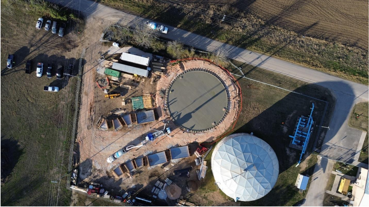
2C – Aerial overhead view of completed concrete pour at Tank Floor Structure.
