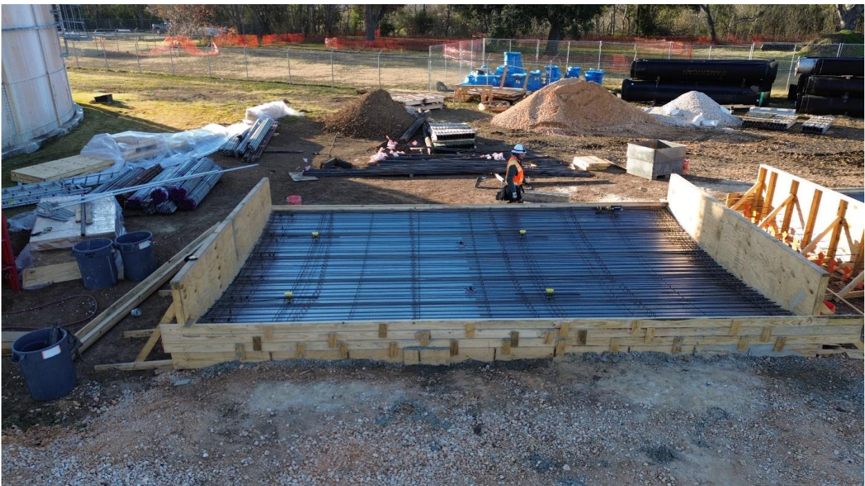
2F – Form with steel panel and reinforcing steel for casting of Wall Panel.
