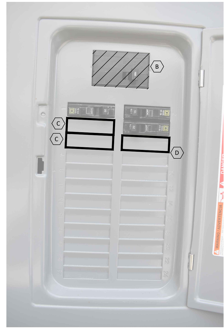
EXISTING GENERATOR ENCLOSURE SUBPANEL
