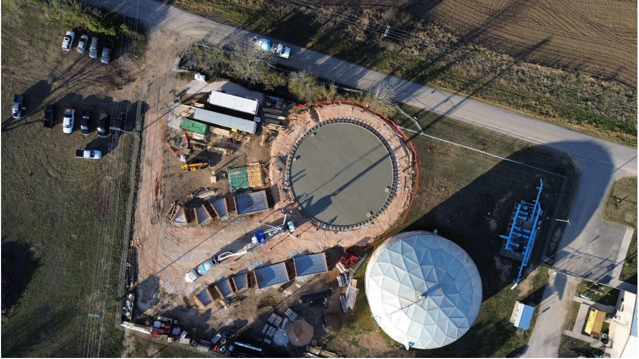
2C – Aerial overhead view of completed concrete pour at Tank Floor Structure.
