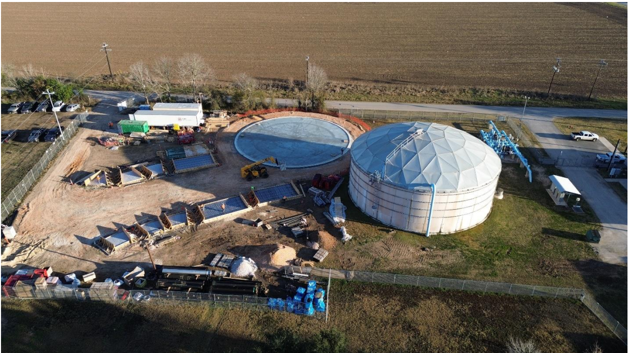
2D – Aerial side view of completed concrete pour at Tank Floor Structure.
