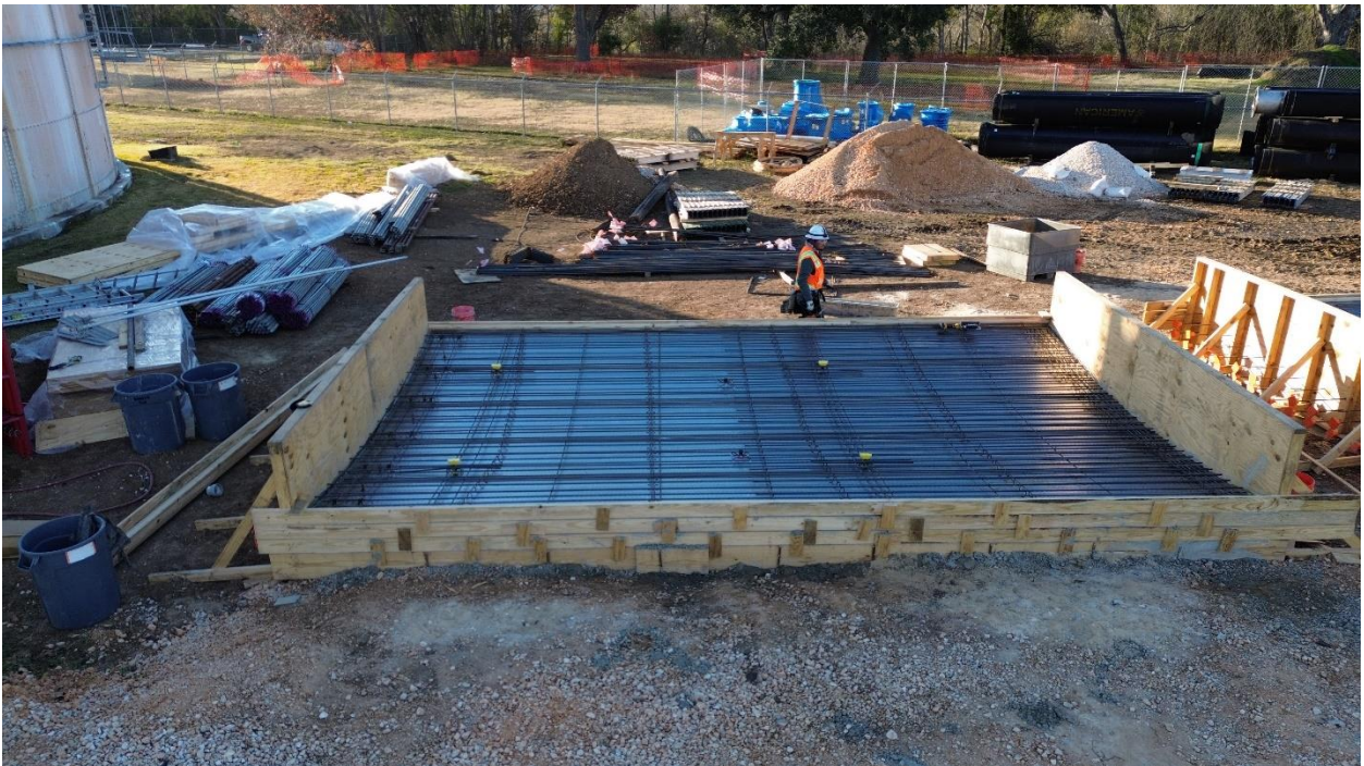
2F – Form with steel panel and reinforcing steel for casting of Wall Panel.
